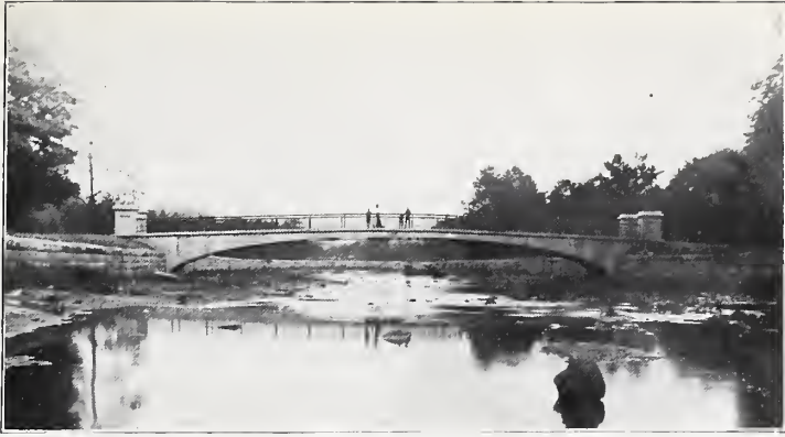
THREE-HINGED CONCRETE ARCH, BROOKSIDE PARK Span Ninety-two Feet. Said to be the Flattest Semi-elliptical Arch of Concrete ever Constructed
